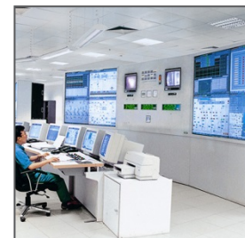
Supervisory Control and Data Acquisition (SCADA)
